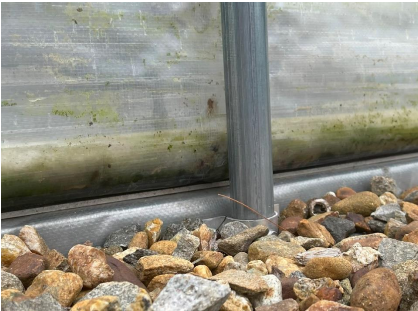
Figure 7. Closeup of seated fabric rail showing adequate but less than complete seal.
